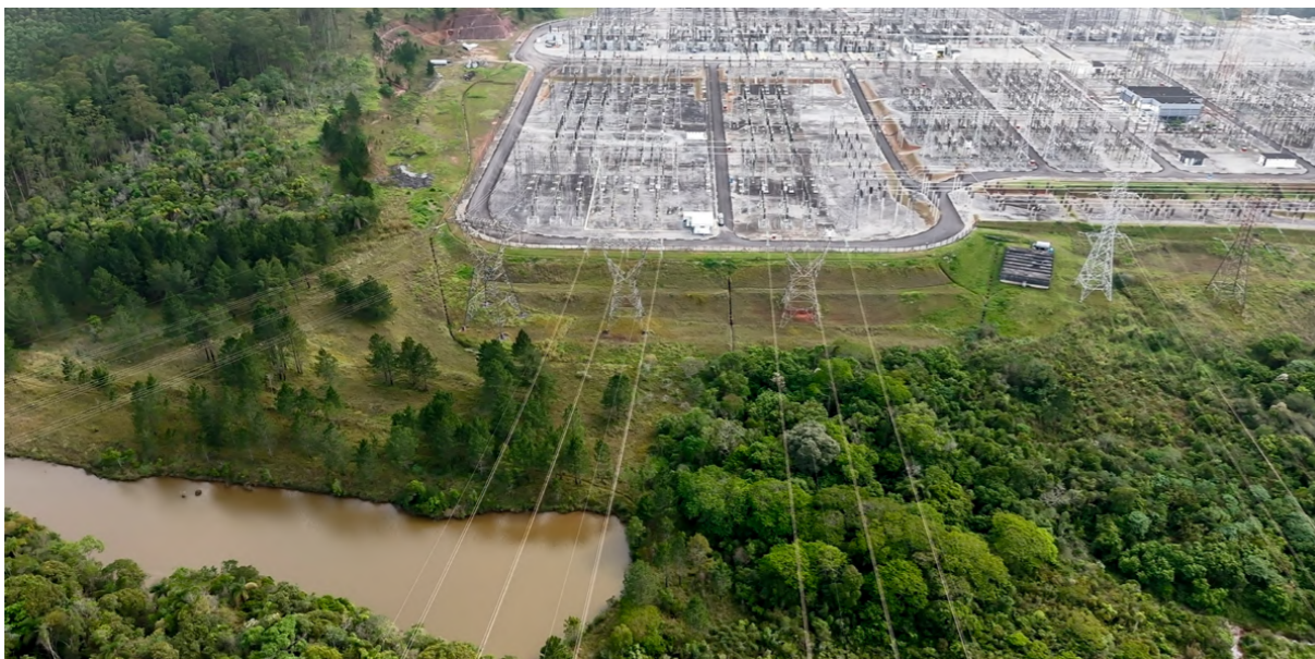
Tijuco Preto substation, Cachoeira Paulista transmission line, Brazil.
