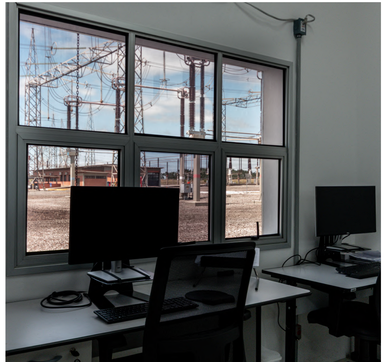
Work center Cachoeria Paulista substation, Brazil.
