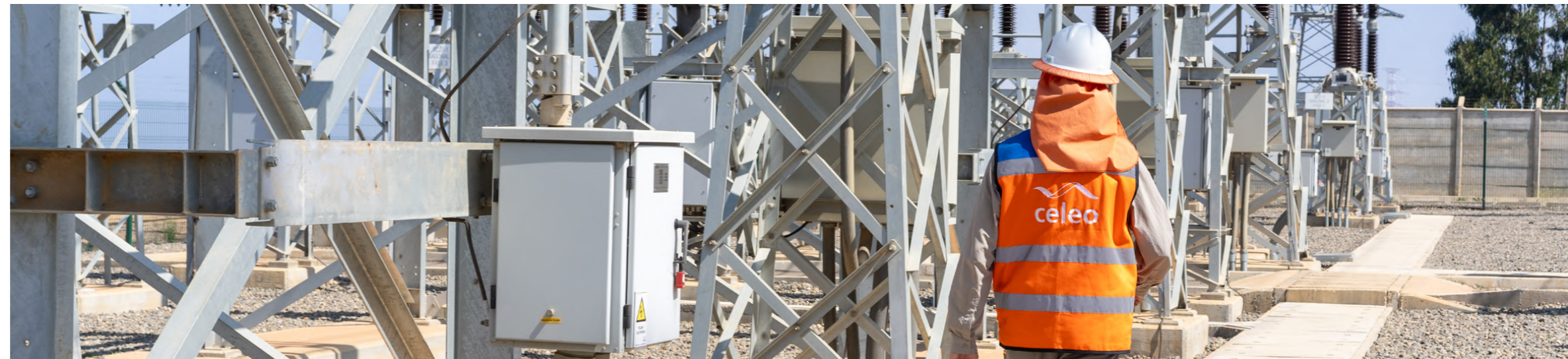
Celeo worker at La Pólvora substation, Chile.
