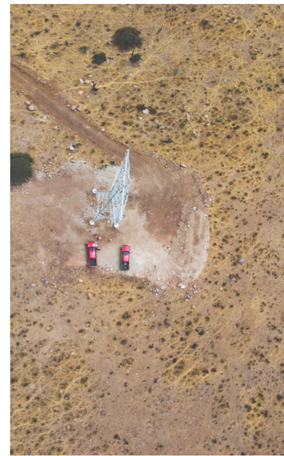
Don Goyo-La Ruca Transmission Line (GOTE), Chile.
