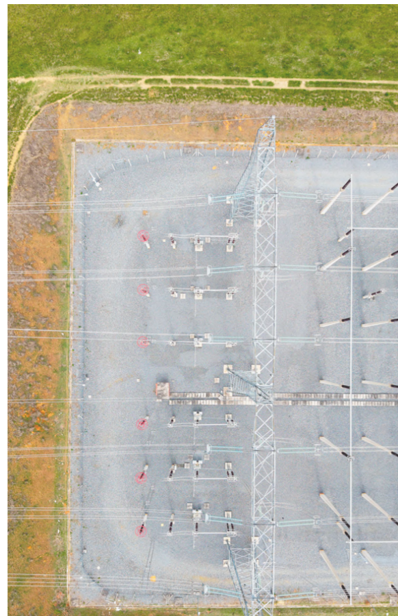
Lorena substation, Cachoeira Paulista transmission line, Brazil.
