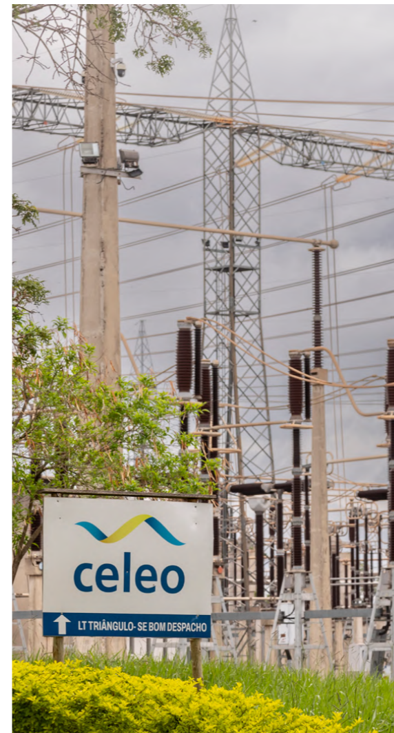
Entrance to the Bom Despacho substation, Triângulo transmission line, Brazil.
