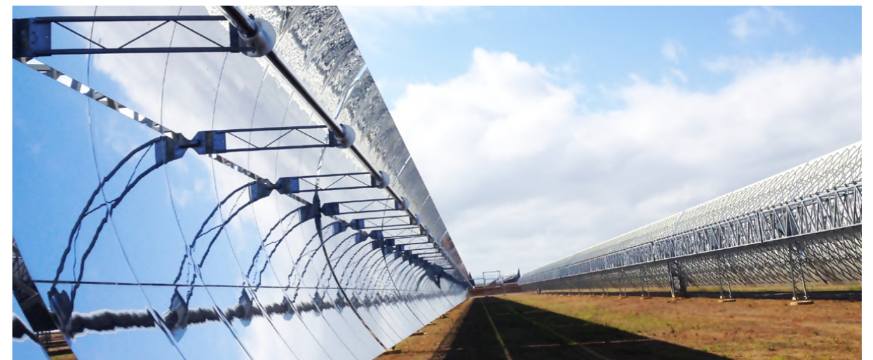
Astexol-2 solar thermal plant, Spain.
