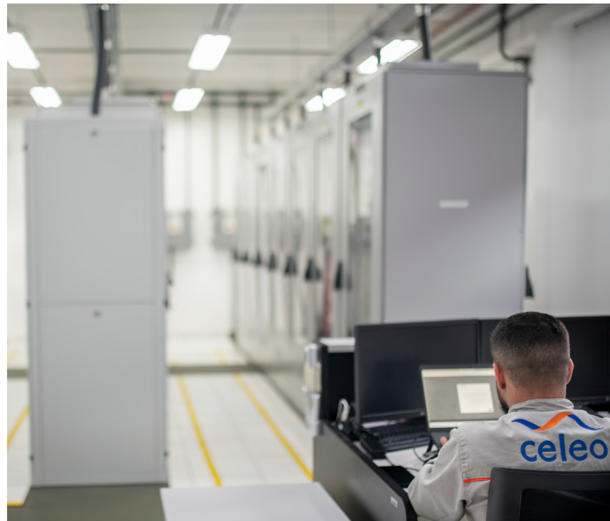
Celeo worker at Fernão Dias substation, Cantareira transmission line, Brazil.
