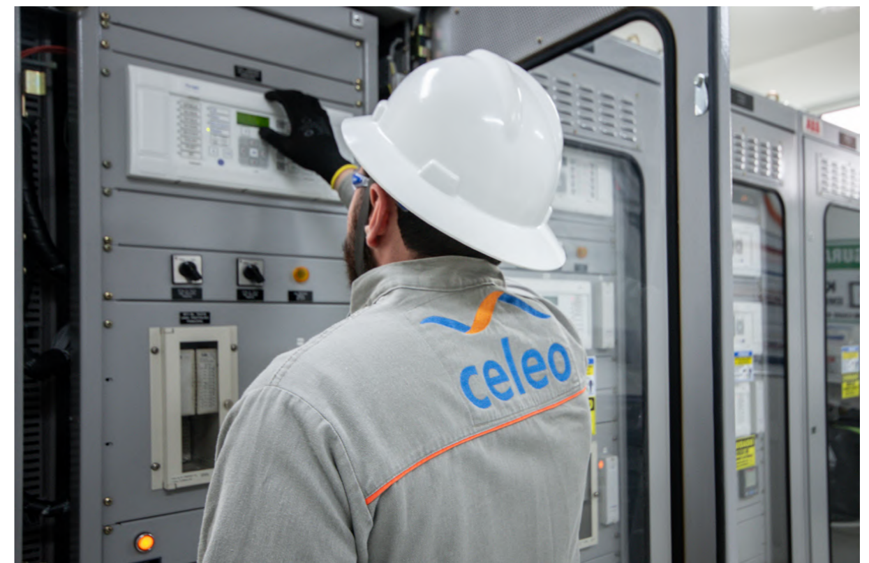
Celeo worker at the control center of the Cachoeria Paulista substation, Brazil.
