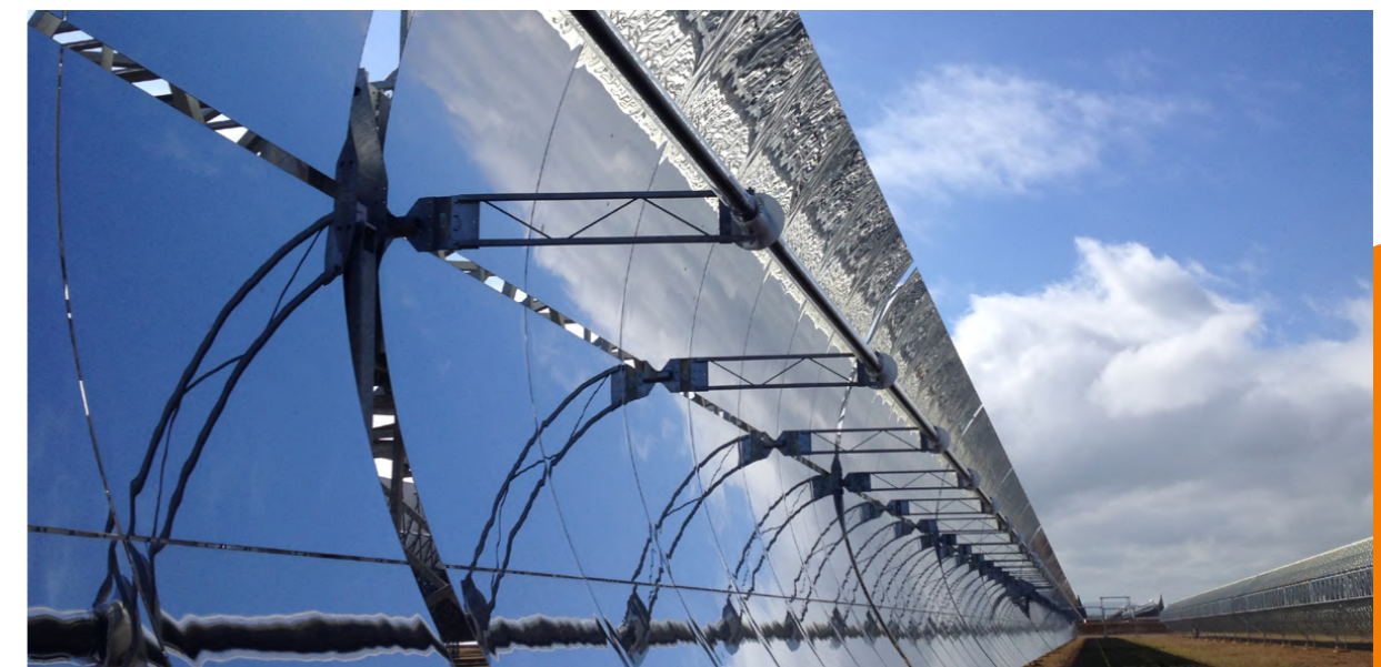
Astexol-2 solar thermal plant, Spain.
